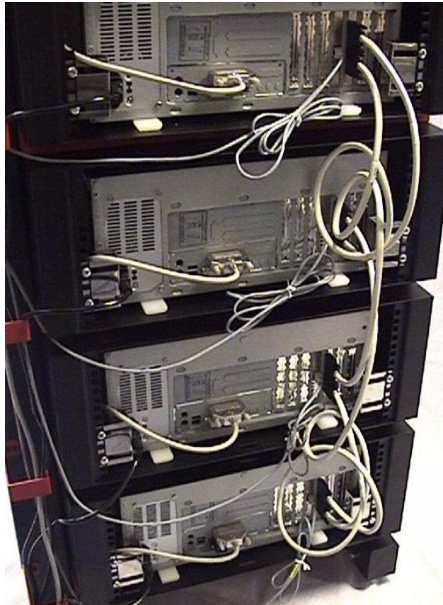
Figure E-17: SCI ring topology cabling on a real system
